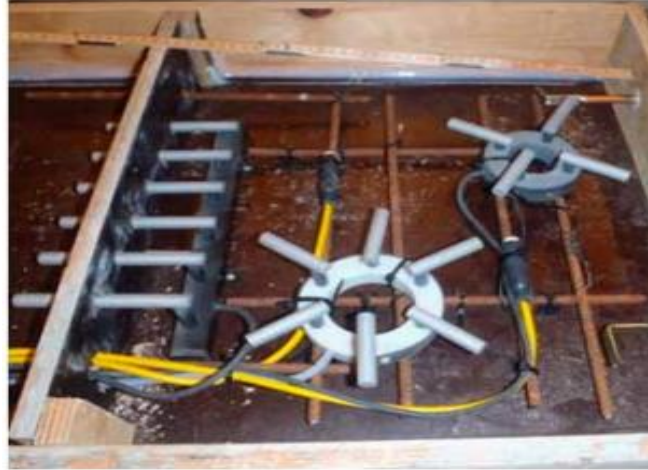
Figure 4-2: Anode probes (set of 4 and set of 6 anodes) installed before concrete casting.
